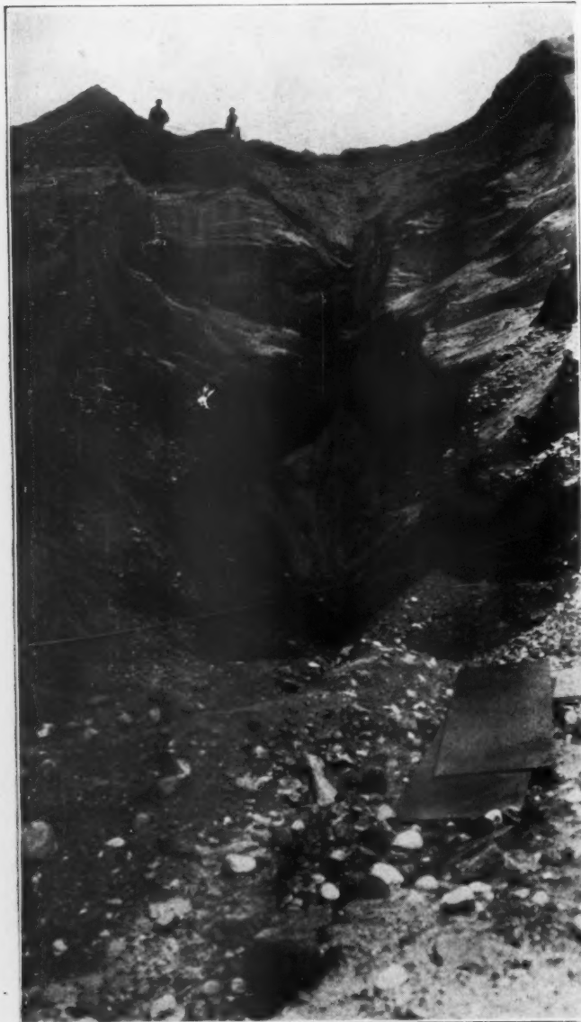
View of Gravel Bank Showing Drag Line Scraper Digging Out a Path at Cloutier and Company
